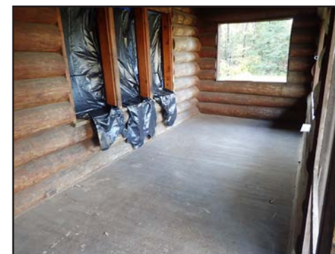
Porch Floor - Before
