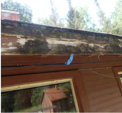
Fascia Board- Before
