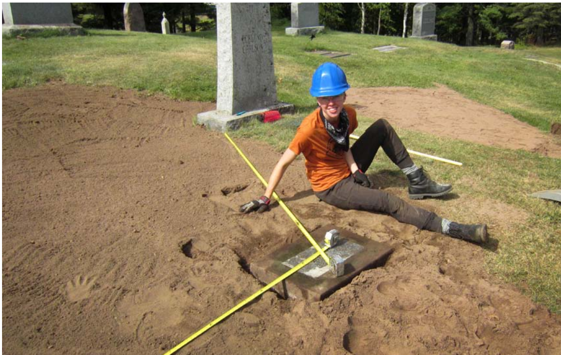
Corpsmember Ashley Brey resets a grave marker at Hillside after re-grading the area to improve future maintenance.
