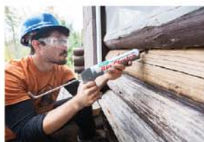
Prairie Portage - Superior National Forest: Crew leader Josh Preston applies caulking to prevent water leaks.
