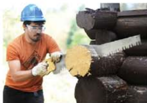
Prairie Portage - Superior National Forest: Josh Preston uses a cross cut saw to shorten logs not protected by the roofline to prevent further damage .
