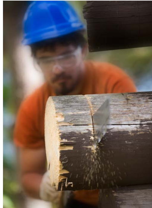
Crew leader Josh Preston removes a log end on the Prairie Portage Cabin to reduce the chance of future rot.
