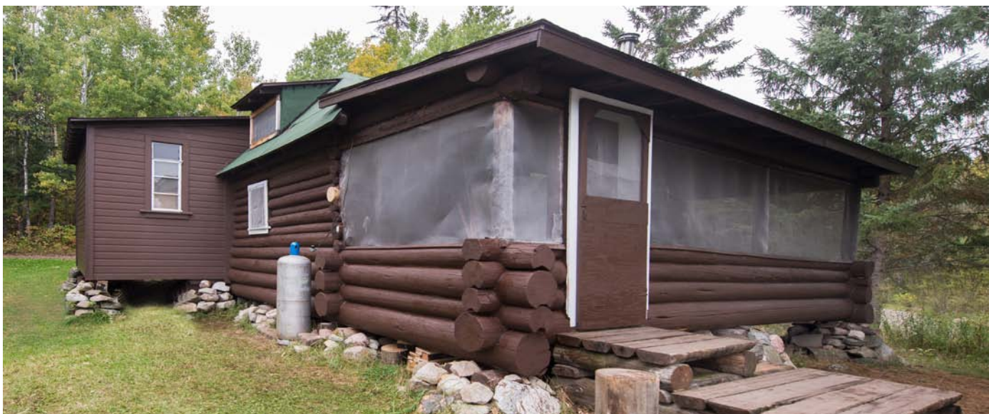
The Prairie Portage Cabin as it stood after a week's work performed by Northern Bedrock and specialists from the U.S. Forest Service.
