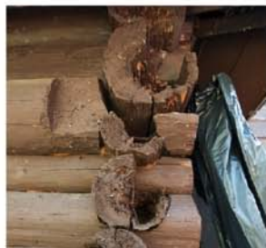
Prairie Portage - Superior National Forest: Decayed logs awaiting plugs and epoxy to stabilize the structure and prevent stop further damage.
