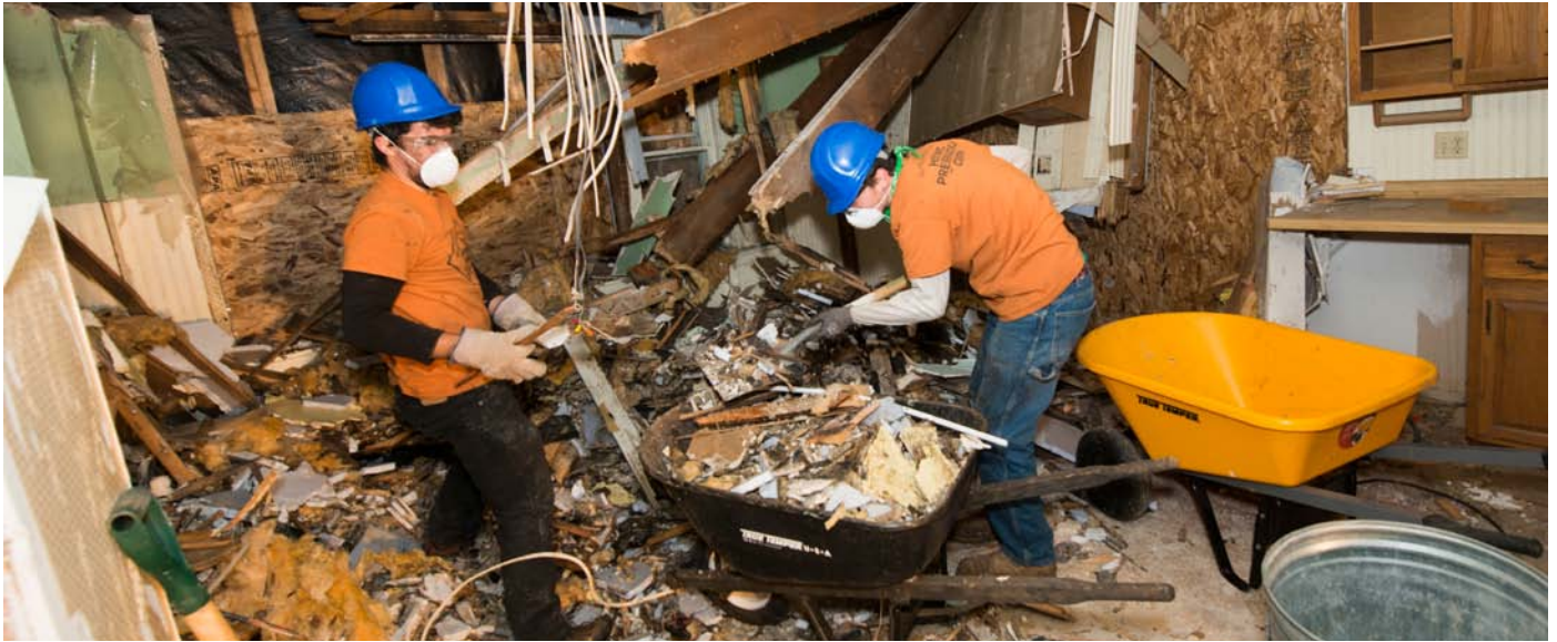
Corpsmembers Josh Preston and Zach Wilson clean up debris in the Rev. Boutwell House after its partial demolition.
