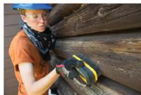
Prairie Portage - Superior National Forest: Crew member Ashley Bray prepares the log's surface with a wire brush, sloughing off loose bits of old stain to accept a new coat of stain.
