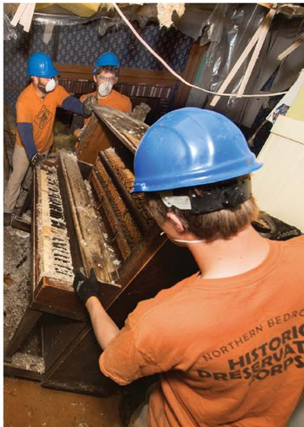
Rev. Boutwell House: Bonk (far left), Preston, and Larson (front) move a piano that had been left in the home during demo.
