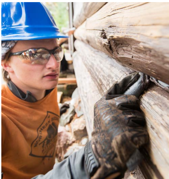
Ryan Larson patiently smooths caulk over the backing rod between gaps in the logs at Prairie Portage cabin.
