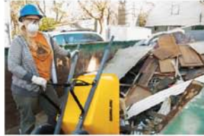
Rev. Boutwell House: Collins transports debris that has been sitting in the home since January.
