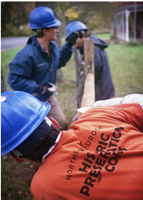
Crew members work together to install new fence outside the Hay Lake School in Scandia, MN.
