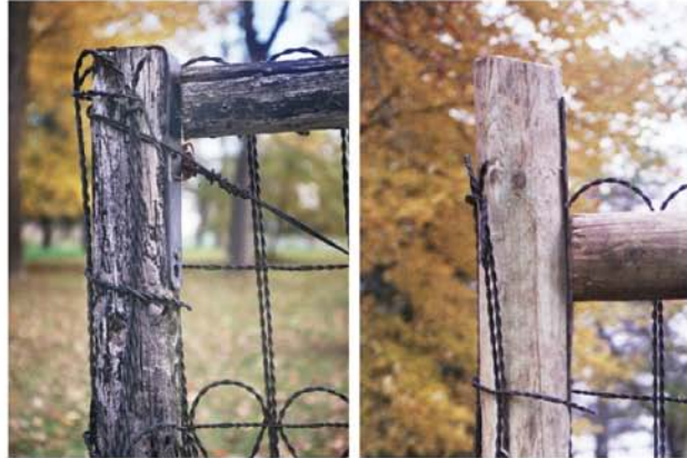
Hay Lake School & Erickson Log Cabin: Fence post before (left) and after (right). Replacing the posts and support logs will ensure the fence remains standing for another two decades.
