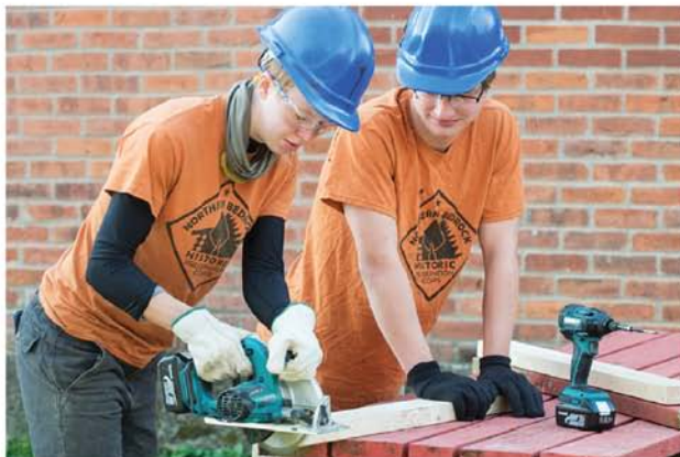
Hay Lake School & Erickson Log Cabin: Crew members Brey and Larson cut new supports to repair the picnic tables on site.
