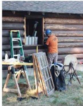
Lac La Croix - Superior National Forest-- Peter Bonk works to scrape old stain off logs. In the foreground is a sharpening wheel for the hand tools needed for historic preservation work and windows awaiting reglazing.
