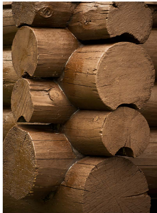
Log ends of the Prairie Portage Cabin after repair and a coat of oil based stain.
