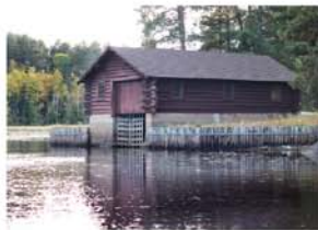
Lac La Croix - Superior National Forest - An after shot of the crew's maintenance work on this rare, drive-in boat house. Because of low water, the corps will return in March to access the front of the boat house via lake ice.
