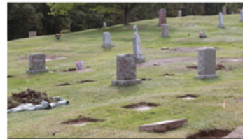
Multiple markers had grass cleared away from them at the Hilltop Cemetery in Carlton last week by Northern Bedrock workers. Some of the stones that have sunk in over the years will be dug up and have fill added underneath them to raise them to level. Jamie.Lund@pinejournal.com
