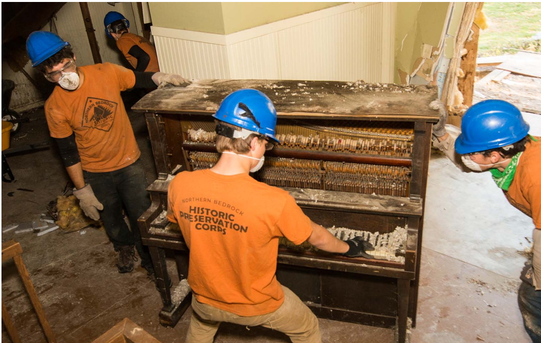
Preston, Larson and Wilson move a piano found in the midst the demolition rubble in the Boutwell House.
