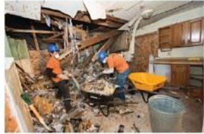
Rev. Boutwell House: Preston and Wilson fill wheelbarrows with debris for removal.
