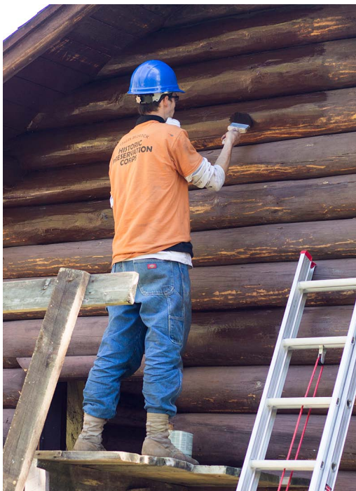
Crew member Wilson applies a coat of oil based stain to the log exterior of the boathouse.
