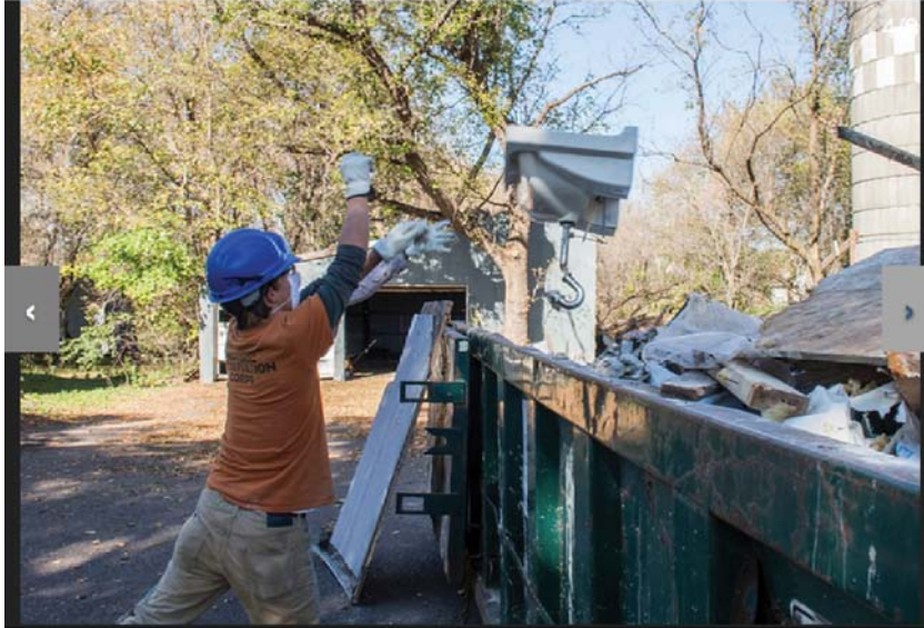
The five-member crew salvaged pieces of the home's original woodwork, but also filled a trash bin with junk. (Pioneer Press: Eric Todd)
