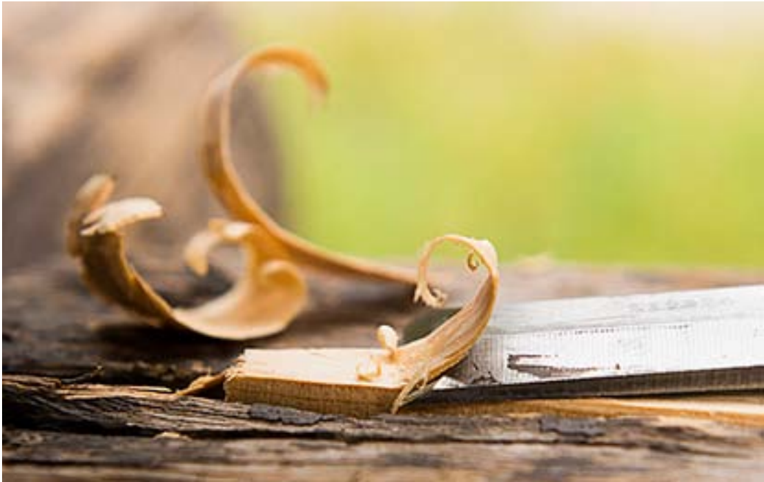
After removing rotted portions of the log, wooden plugs were hand shaped to fit into the logs.
