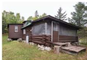
Prairie Portage - Superior National Forest: After the project was caulked, sealed, stained and the door freshly painted, a sense of pride was felt by the crew. They were part of keeping this structure sound for another twenty years.
