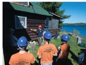
Prairie Portage - Superior National Forest: Lee Johnson, Heritage Program Manager and lead project host, illustrates how the south side of the building has weathered. The crew maintained the structure by installing backing rod, caulking, inserting needed plugs and staining.
