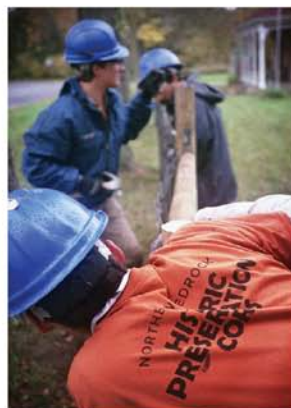
Hay Lake School & Erickson Log Cabin: Crew members Wilson (front), Larson (rear left) and Preston (rear right) work together to install a cross beam on the fence.
