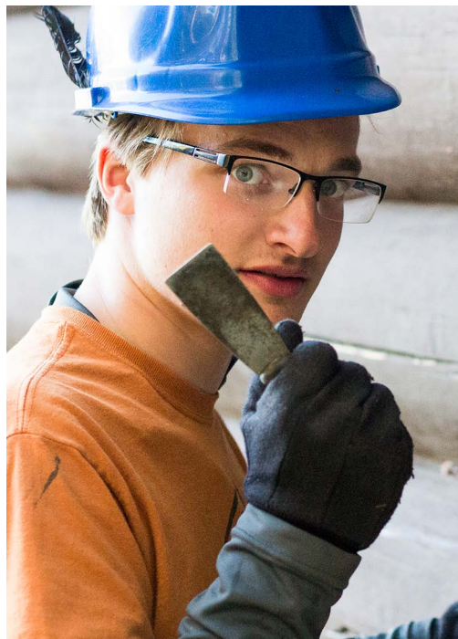
Larson pushes foam backing rod into checks in the log exterior in preparation for sealant and stain.
