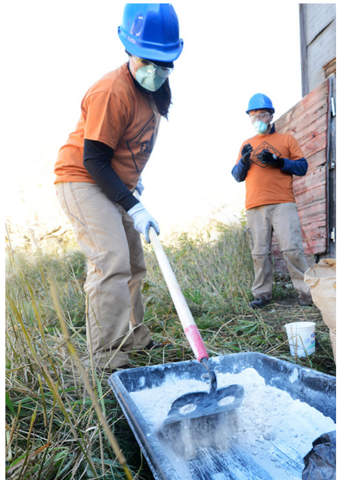
Northern Bedrock crew members Meghan Weber and Zach Small mixing mortar for flooring repairs at the McDougall Barn (Royaltown, MN).
