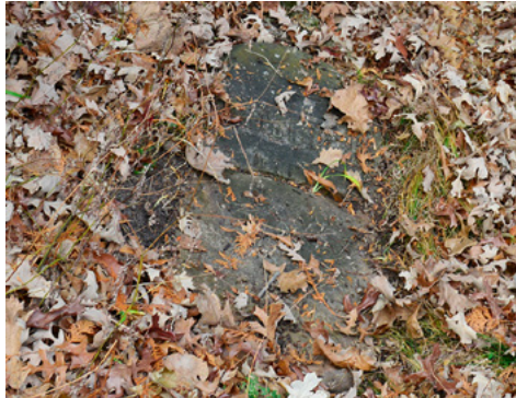
A broken stone monument threatened to be lost by encroaching soil and sod prior to Northern Bedrock's crew cleaning and digging the stone out.
