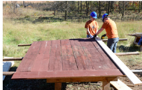
Operations Director Brooke Tappe and Crew Leader Anne Ketz measure the first exterior replacement boards for the second layer of McDougall Barn's east doors.
