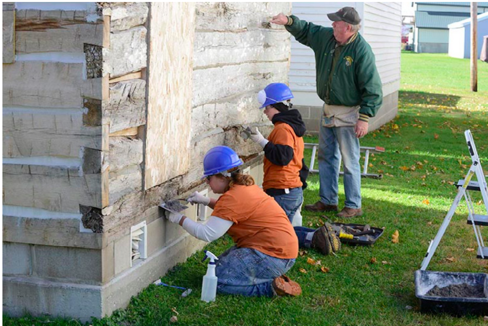
Crew members Lexi Kosik and Jennifer Sustar work with Rushford Historical Society board member Jack O'Donnell on daubing the historic log cabin at the Rushford Depot Museum site in Rushford, MN.
