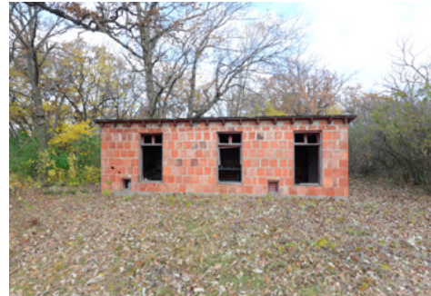
The masonry chicken coop on the McDougall Farmstead site after vegetation removal.
