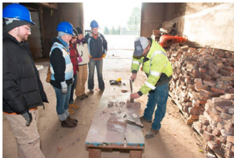
Duluth Armory (Duluth, MN): The crew getting an introduction on brick cleaning techniques from Bricklayer Foreman, Darrell Koffler (from left to right: Zach, Jennifer, Lexi, Meghan, Anne, and Darrell Koffler).
