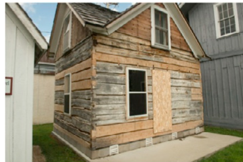
The historic log cabin, acquired by the Rushford Historical Society Museum, the crew will be working on this week.
