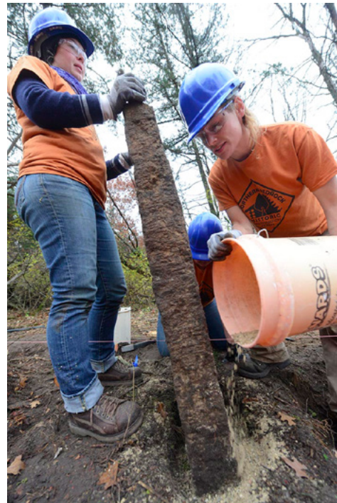
Crew member Jennifer Sustar and Operations Director Brooke Tapp straightening a fallen stone fence post at Oakwood (Sherwood) Cemetery in Rushford Village, MN. Brooke is pouring and tamping
