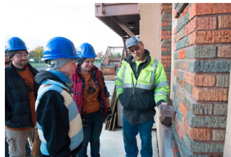
Darrell Koffler, mason foreman for Macpherson Towne, showing the crew the uniqueness of the size and color of the 100 year-old bricks used in the construction of the Duluth Armory (left to right: Zach Small, Jennifer Sustar, Alexandra Kosik, Darrell Koffler).
