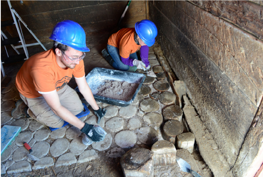
Crew members Zach Small and Jennifer Sustar apply mortar to a horse stall floor in west end of the McDougall Barn.
