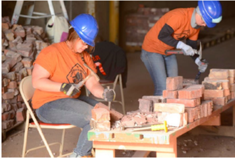
Crew members Alexandra Kosik and Jennifer Sustar hard at work cleaning bricks at the Duluth Armory.
