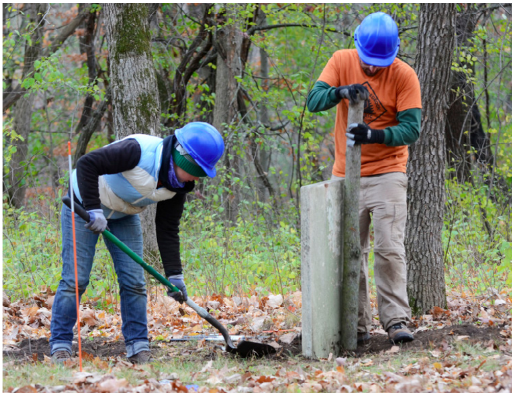
Crew members Jennifer and Zach tamp soil around a newly set stone monument. This monument, along with another reset nearby, had been out of the ground, leaning against a tree, since the 1980s according to Martens.
