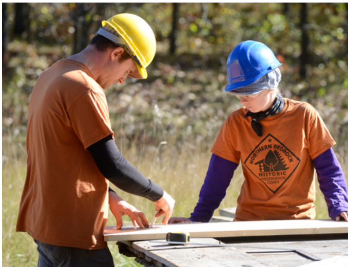
Technical Specialist Adam Valesano working with crew member Jennifer Sustar on repairing the main doors of the McDougall Barn (Royalton, MN).
