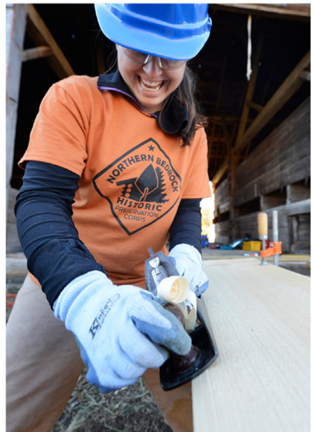
Meghan putting a bevel on a board to match the historic design.
