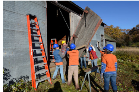
Crew members removing the heavy east doors of McDougall Barn for repairs (visible from left to right: Brooke Tapp, Adam Valesano, Zach Small, Lexi Kosik, Meghan Weber, Jennifer Sustar).
