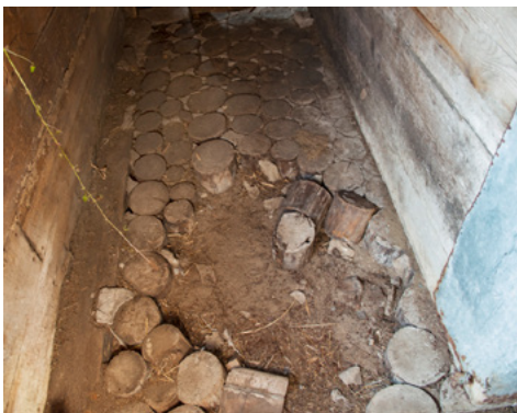
Horse stall floor, east end of the McDougall Barn, prior to repairs.
