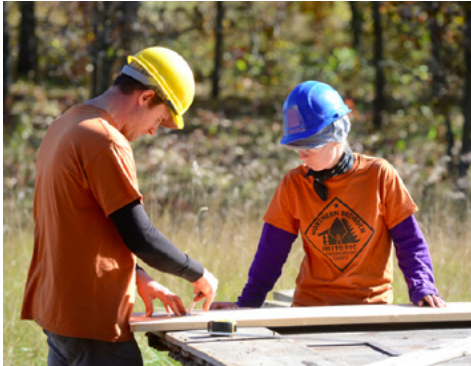
Jennifer Sustar works with technical specialist Adam Valesano in measuring and cutting replacement boards for the east doors of the McDougall Barn.
