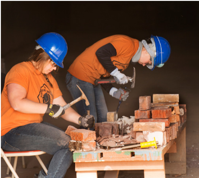
Northern Bedrock crew members Jennifer Sustar and Alexandra Kosik cleaning bricks at the Duluth Armory (Duluth, MN).
