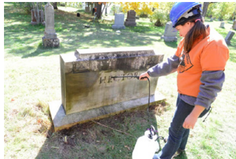
Stone cleaning in progress by crew member Meghan Weber at Scandia Cemetery.
