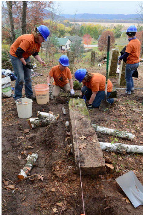
Crew Leader Anne Ketz, Operations Director Brooke Tapp and crew members Lexi Kosik and Jennifer Sustar working on resetting a fallen stone fence post at Oakwood (Sherwood) Cemetery in Rushford
