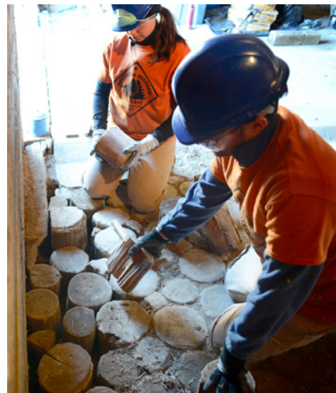
Crew members Meghan Weber and Jennifer Sustar installing mortar in the flooring of the west-end horse stall in the McDougall Barn.
