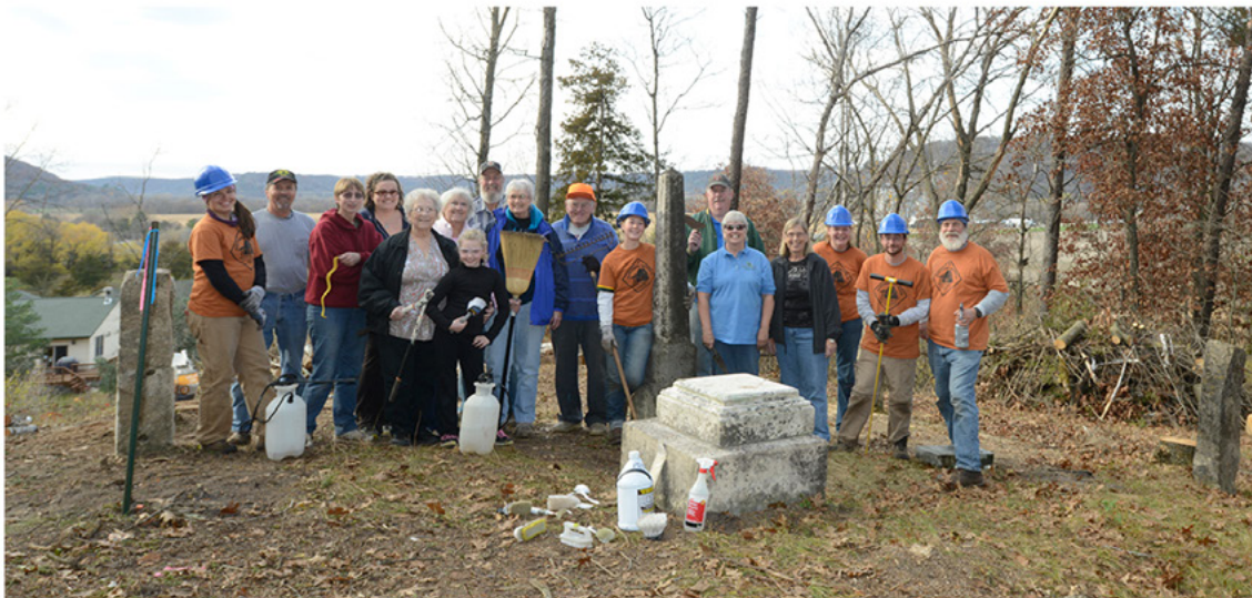
The crew trains a group of 15 people in stone cleaning and resetting techniques.
