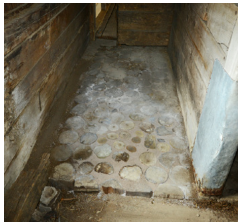
Horse stall floor, east end of the McDougall Barn, after repairs were completed by the Northern Bedrock crew.
