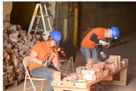
Duluth Armory (Duluth, MN): Crew members Lexi and Jennifer work on cleaning mortar off of 100 year old bricks for reuse in the Armory restoration.
