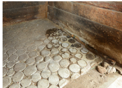
Horse stall floor, west end of McDougall Barn, after repairs by the Northern Bedrock crew.
