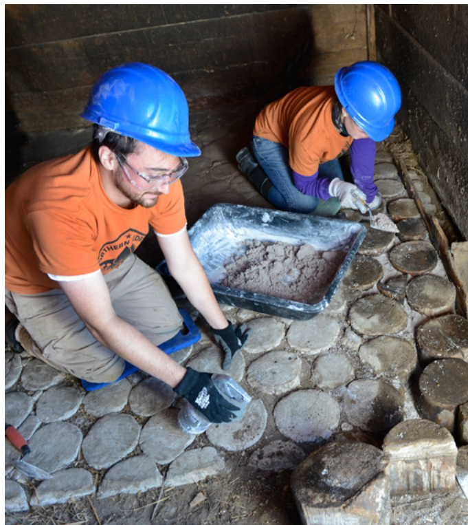
Crew members Zach Small and Jennifer Sustar resetting the end-grain floor in McDougall Barn (Royalton, MN).
