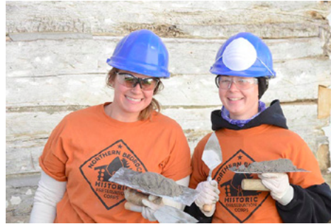
Lexi Kosik and Jennifer Sustar posing in front of the log cabin at the Rushford Depot site in Rushford, MN, with the lime and sand based mortar used in daubing the exterior logs.
