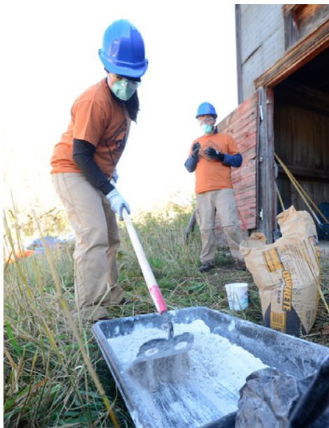
Crew members Meghan Weber and Zach Small mixing lime mortar for installation in the McDougall Barn horse stall floors.
