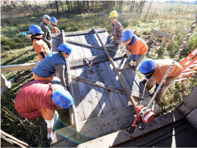
Northern Bedrock crew, staff and Technical Specialists Paul Ormseth and Adam Valesano, removing a barn door for repairs at the McDougall Barn (Royalton, MN).
