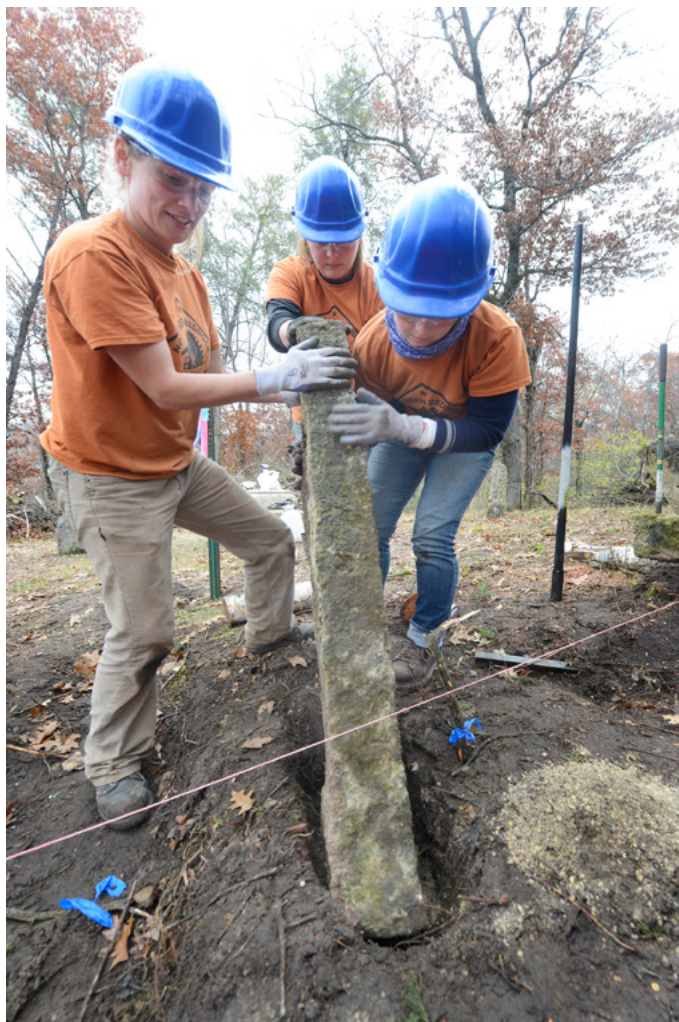
Northern Bedrock Operations Director Brooke Tapp assisting crew leader Anne Ketz and crew member Jennifer Sustar in resetting a stone fence post at Oakwood Cemetery (Rushford, MN).
