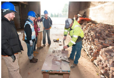
Crew members learning how to clean mortar off bricks for reuse (left to right: Zach Small, Jennifer Sustar, Alexandra Kosik, Meghan Weber, Anne Ketz and Darrell Koffler, foreman for Macpherson Towne).
