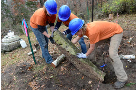
Anne Ketz, Jennifer Sustar and Brooke Tapp lifting into place one of the fallen stone fence posts to be reset in the ground at the Oakwood (Sherwood) Cemetery in Rushford Village, MN.
