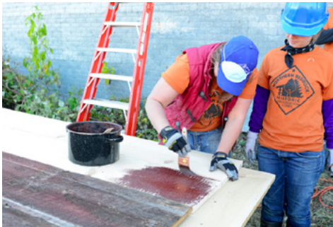
Jennifer Sustar looks on Lexi Kosik spreads the freshly mixed linseed oil based paint on the replacement boards in the first exterior layer of McDougall Barn's east doors.
