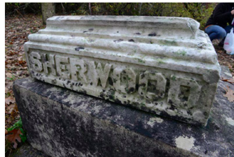
The base of the Sherwood obelisk monument after cleaning at the Oakwood (Sherwood) Cemetery in Rushford, MN. The black fungus growing on this monument was especially difficult to remove but the D2 Biological Cleaner used on the stone will keep working over time to kill the growth and clean the stone.
