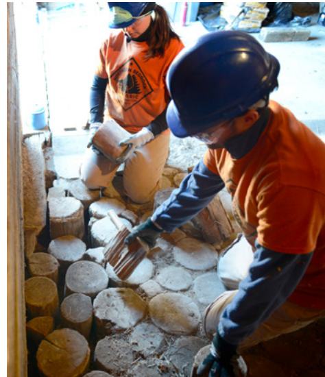
McDougall Barn (Royalton, MN): Crew members Meghan and Zach working on resetting the end-grain log flooring in the barn's horse stalls.
