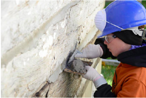
Jennifer Sustar concentrating on placing daubing mortar in between the logs in the historic log cabin at the Rushford Depot site in Rushford, MN.
