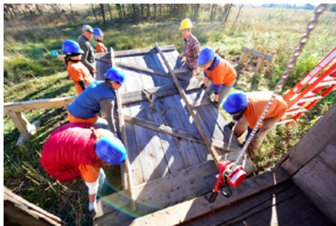
One of the 7' by 12' east doors of McDougall Barn being lifted by crew members with the help of onsite technical specialists Paul Ormseth and Adam Valesano. (From left to right: Lexi Kosik, Brooke Tapp, Meghan Weber, Paul Ormseth, Jennifer Sustar, Adam Valesano, Anne Ketz, and Zach Small).
