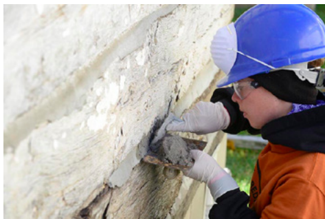
Jennifer Sustar concentrating on placing daubing mortar in between the logs in the historic log cabin at the Rushford Depot site in Rushford, MN.
