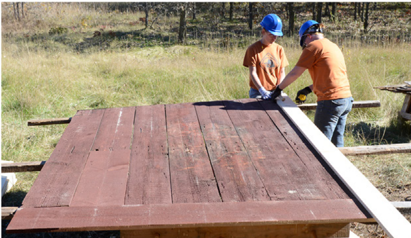
Brooke & Anne measuring replacement boards for the outer layer of the door.
