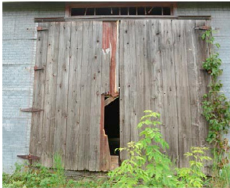
Two 7' by 12' east doors of the McDougall Barn prior to repairs by the Northern Bedrock crew.
