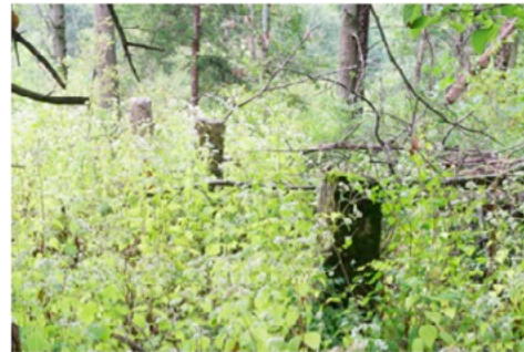
Stone fence posts needing cleaning and resetting in Oakwood (Sherwood) Cemetery.
