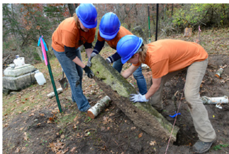
Oakwood (Sherwood) Cemetery (Rushford, MN): Crew leader Anne with crew member Jennifer and Operations Director Brooke lifting a stone fence post
