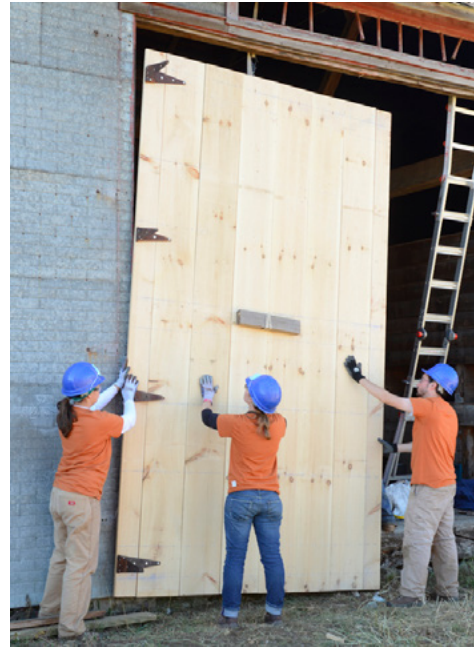
One of the east doors of the McDougall Barn being hoisted into place for reinstallation after repairs (from left to right: Meghan Weber, Jennifer Sustar, and Zach Small).
