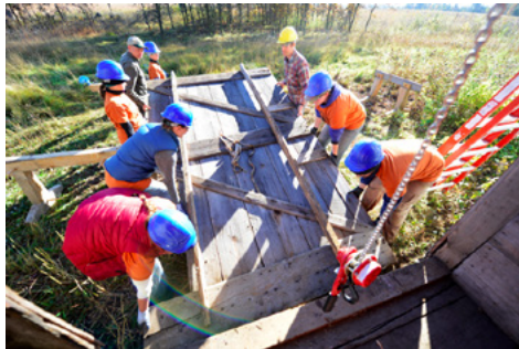
McDougall Barn (Royalton, MN): The crew working together with technical specialists Adam Valesano and Paul Ormseth, to lower the large east side barn doors for repairs (from left to right: Lexi, Brooke, Meghan, Paul Ormseth, Jennifer, Adam Valesano, Anne, and Zach).
