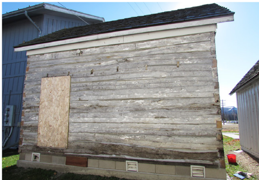
The crew finishes the chinking and daubing on the north side of the cabin.
