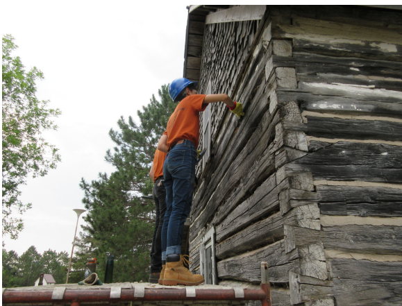
Corpsmembers use scaffolding to access the gable wall of a pioneer cabin to replace the mortar daubing.
