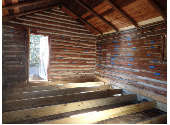
Floor joists being installed. The wall to be rechinked is visible on the right.
