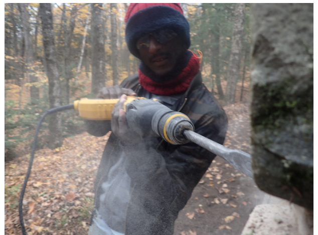
Franklin Lake - An Americorps volunteer does some of the 'heavy lifting' of removing mortar with a rotary hammer.
