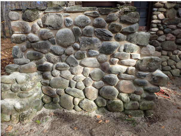
Franklin Lake - The above wall finished with mortar repointed and certain areas rebuilt.
