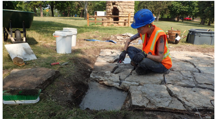
The table pads were made of limestone set in a bed of mortar on top of a concrete foundation. Loose or missing stones were replaced with salvaged material.
