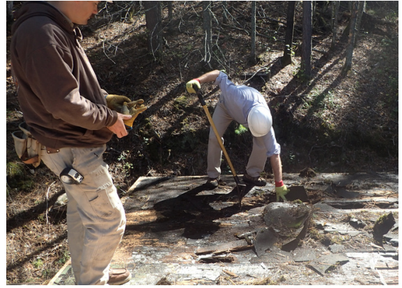
The accumulation of bio-growth on the bathroom lead the complete deterioration of the roof structure. Here a volunteer and staff removes the failed material.
