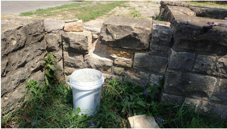
The overlook wall at Graeser Park shows signs of deterioration since its construction in the 1930s
