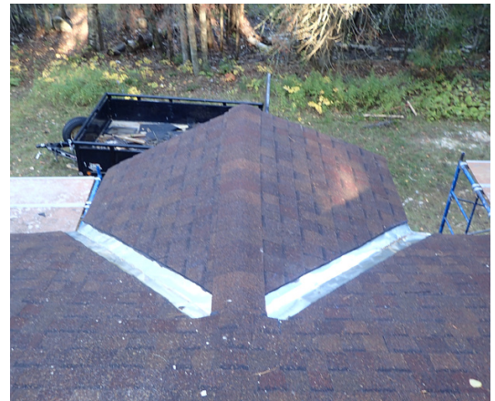
Keeping with the original materials and execution, valley flashing was made with galvanized steel and left exposed.
