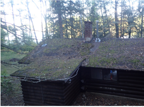
The east elevation showing heavy accumulation of duff and moss.
