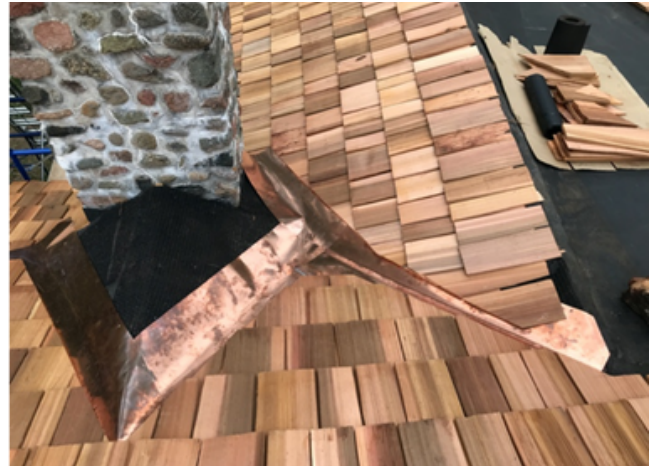
The chimney crickets were flashed with copper and then cedar shakes installed.
