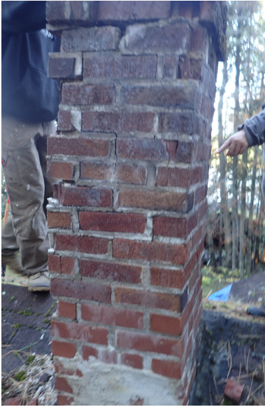
The chimney proved to be so deteriorated that most brick was unsalvageable and needed complete rebuilding.
