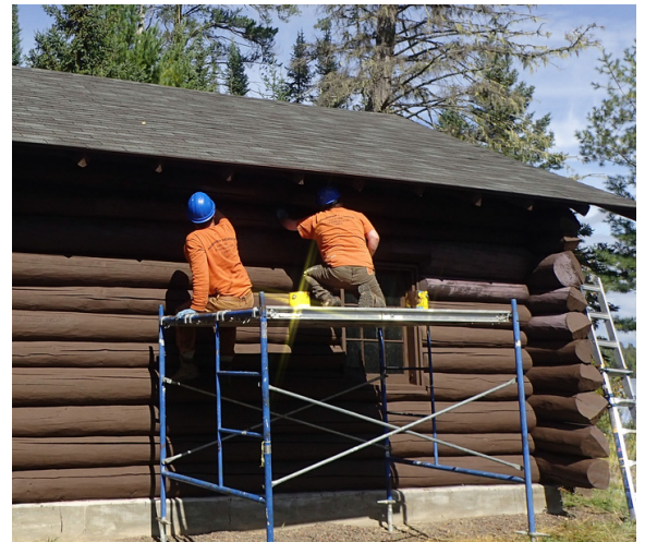
Members staining under the lintels of the guard station.
