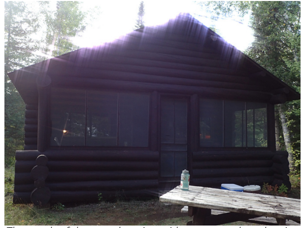
The porch of the guard station with some weathered stain.
