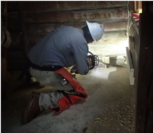
Using a chain saw, a staff member cuts a slot to the wall to be pinned and then hydraulically lifted.
