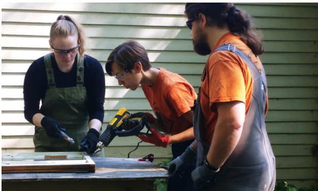
Northern Bedrock crew members show how to safely and effectively remove old glazing compound.
