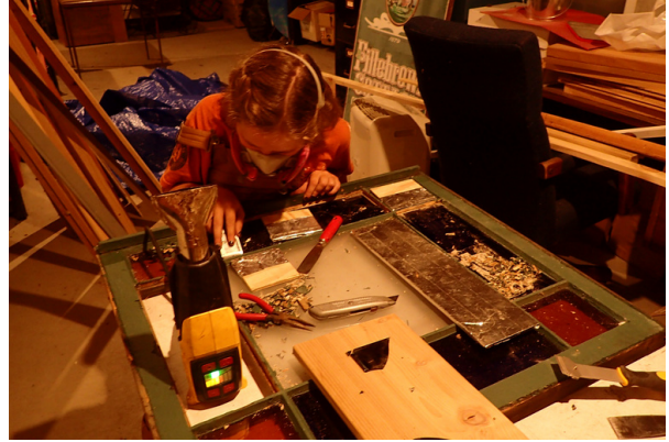
Restoration work on the windows at Fillebrown involved the careful cleaning of original stained glass.
