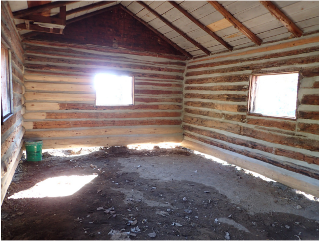
Interior of the Kettle Falls Tender's Cabin without a floor. Note some log replacement has been previously done.
