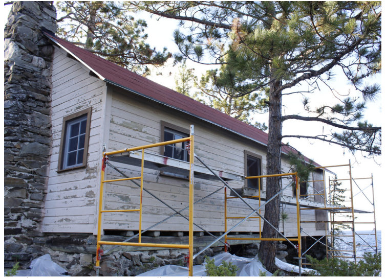
The entire eastern eave wall needed staging erected, this was two or three courses tall for the majority.
