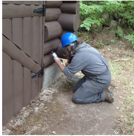
A Corpsmember packs checks with close cell foam prior to sealing with caulk.
