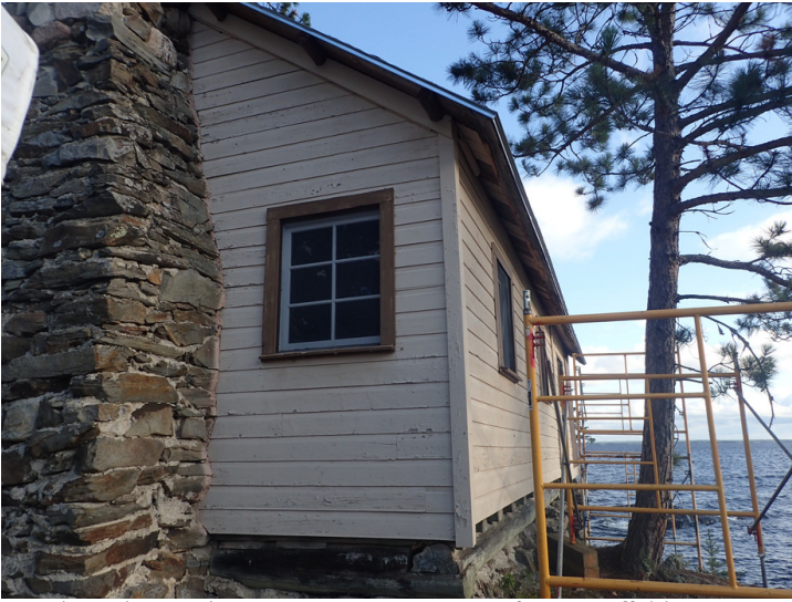
The Polariss Cabin at Camp Marston, significant scaffolding was needed to gain access to one gable walls and one eave wall.
