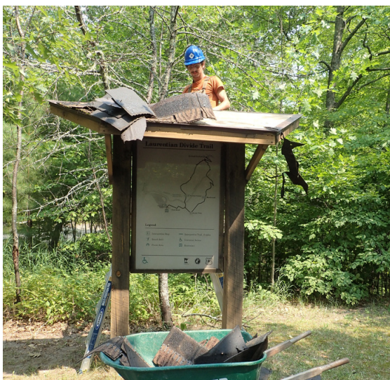
Removing the failed roof covering on one of the information kiosks at the Wayside
