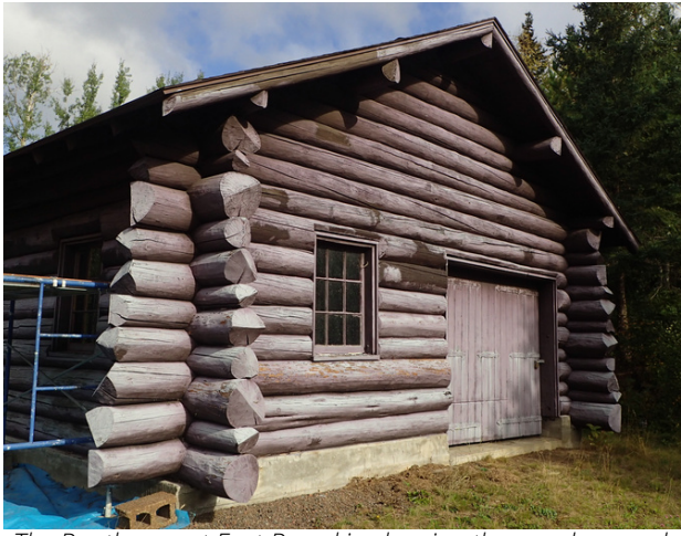
The Boathouse at East Bearskin showing the sun damaged, originally Oxford brown, stain.
