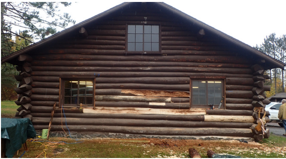
Rotten bits of logs have been removed on this wall at Isabella Work Station.
