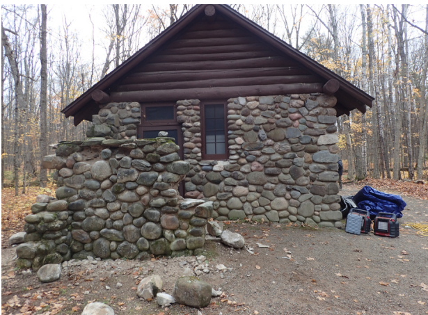
Franklin Lake - Rocks that came out during chiseling were kept in their general locations so as to keep track when rebuilding.
