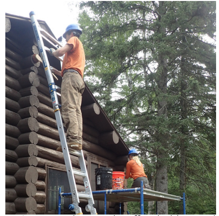
Corpsmembers and staff us ladders and scaffolding to access the gable wall and roof overhang.
