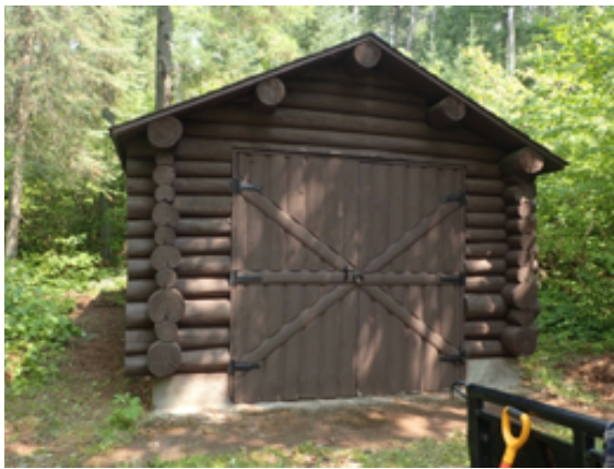
Boathouse before exterior refinishing and removal of accumulated sediment
