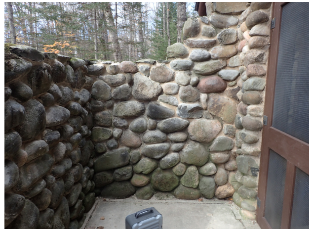
Franklin Lake - Using a milk room heater helped the Natural Hydraulic Lime based mortar to set despite the cold temperatures .
