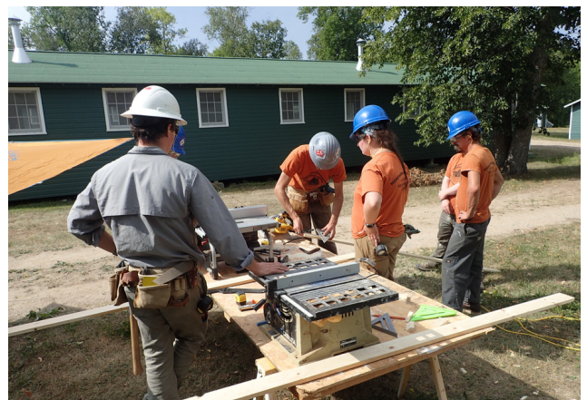
Corpsmembers learn how to replicate missing trim elements from the Recreation Hall.
