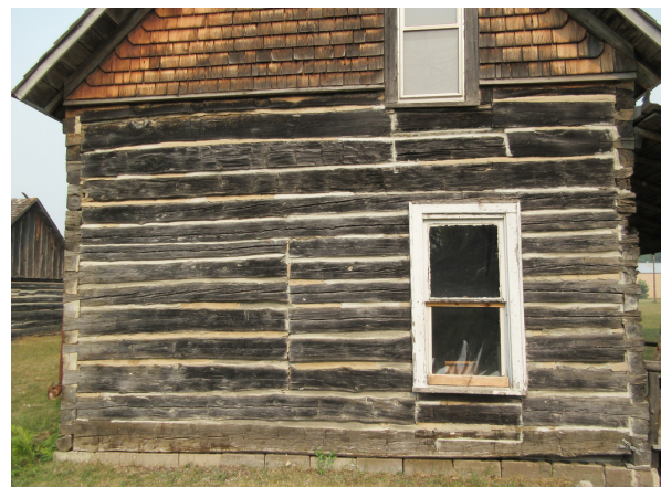
The same gable wall as the photo at right, after daubing replacement.
