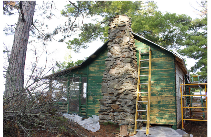
The surface was lightly scuffed prior to priming with an oil based primer and two finish coats of latex paint.
