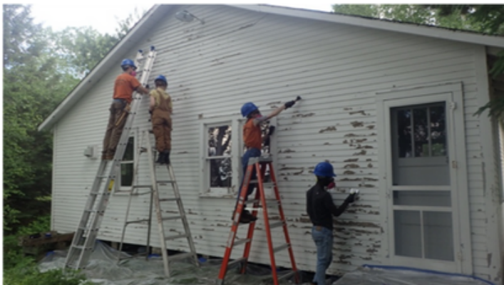
Corpsmembers us a variety of ladders to gain access to entire wall surface.
