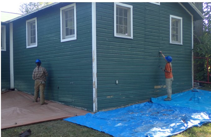
AmeriCorps volunteers scrape the exterior of the east wing of the Education Building.
