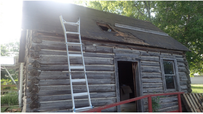
The Becker County Fairground Cabin between removing the failed roof covering and installing the new cedar shingles.
