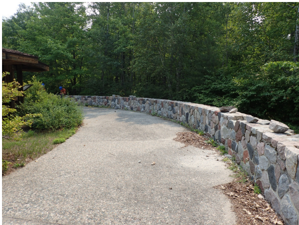
The main overlook wall prior to restoration, note the stone that rest on top of the wall since they have fallen out.
