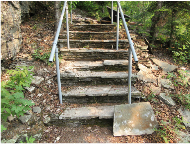
An example of the masonry stairs along the Mt. Rose trail prior to restoration work.
