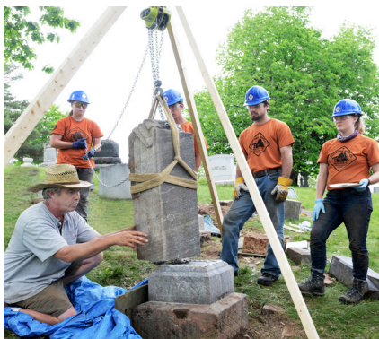
Jonathan Appell using a chain hoist to set a monument onto the base
